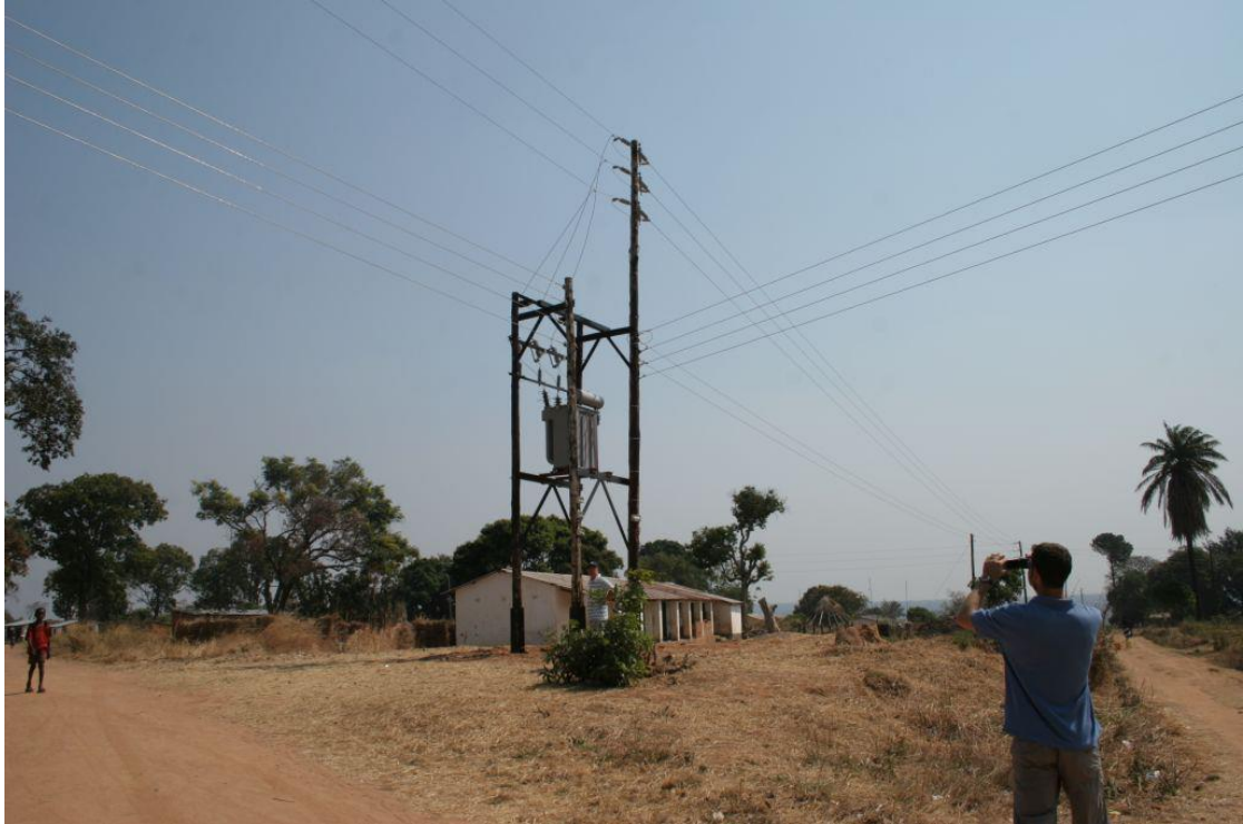
(a) Transformer under medium-voltage line, spanning low-voltage trunk network
